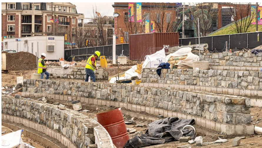
RASH FIELD PARK 2 continued to rise between Key Highway and the Inner Harbor in March as construction crews started to build some of the park's central structures. The concrete base of the multiuse "Fieldhouse" was poured (top photo) and the tiered "Amphitheater" seating (above) that will look out over "The Lawn" toward the harbor took shape. Construction on the new park began with a groundbreaking in April 2025 and is expected to be complete by the end of this summer with opening day in the fall. Photos by Mary Braman.
